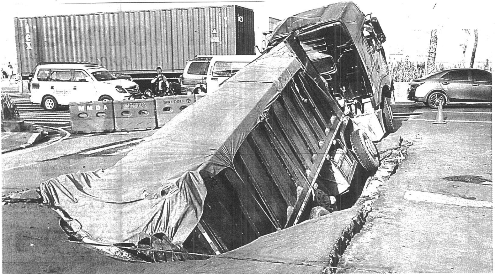
Sinkhole? Not really – just a drainage box destroyed by an overloaded truck carrying Pampanga sand bound for Manila Bay's beach.
