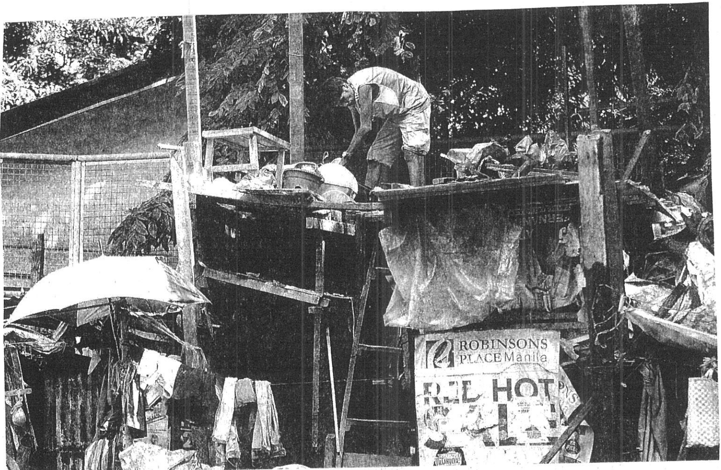
SHANTIES NO MORE. Workers from the Pasig River Rehabilitation Commission demolish shanties along Estero Magdalena on Claro M. Recto Avenue in Manila's Binondo district Thursday. About 270 families will be relocated to Trece Martirez, Cavite. The clearing operation is in preparation for the coming rainy season to declog the flow of the Pasig River. Norman Cruz
