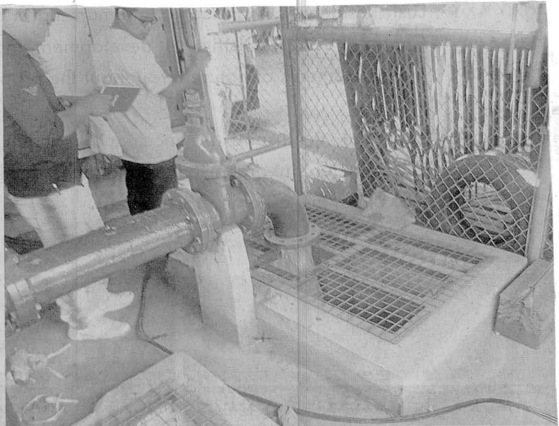
DEEP WELL IN ANTIPOLO CITY The National Water Resources Board has allowed Manila Water to reopen deep wells that have been ordered closed and to drill new ones to help ease water shortage in Metro Manila. —PHOTO COURTESY OF MANILA WATER
