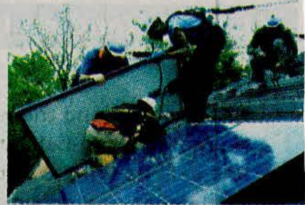
SOLAR power panels installation training for women is life-changing skills that benefit the whole community, and reduce the impact on the environment. AFP
